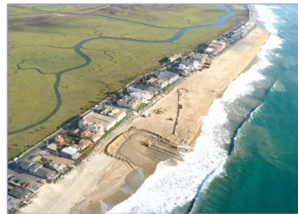
Figure 27. Beach Nourishment in Imperial Beach in 2012 as part of SANDAG's Regional Beach Sand Project II
